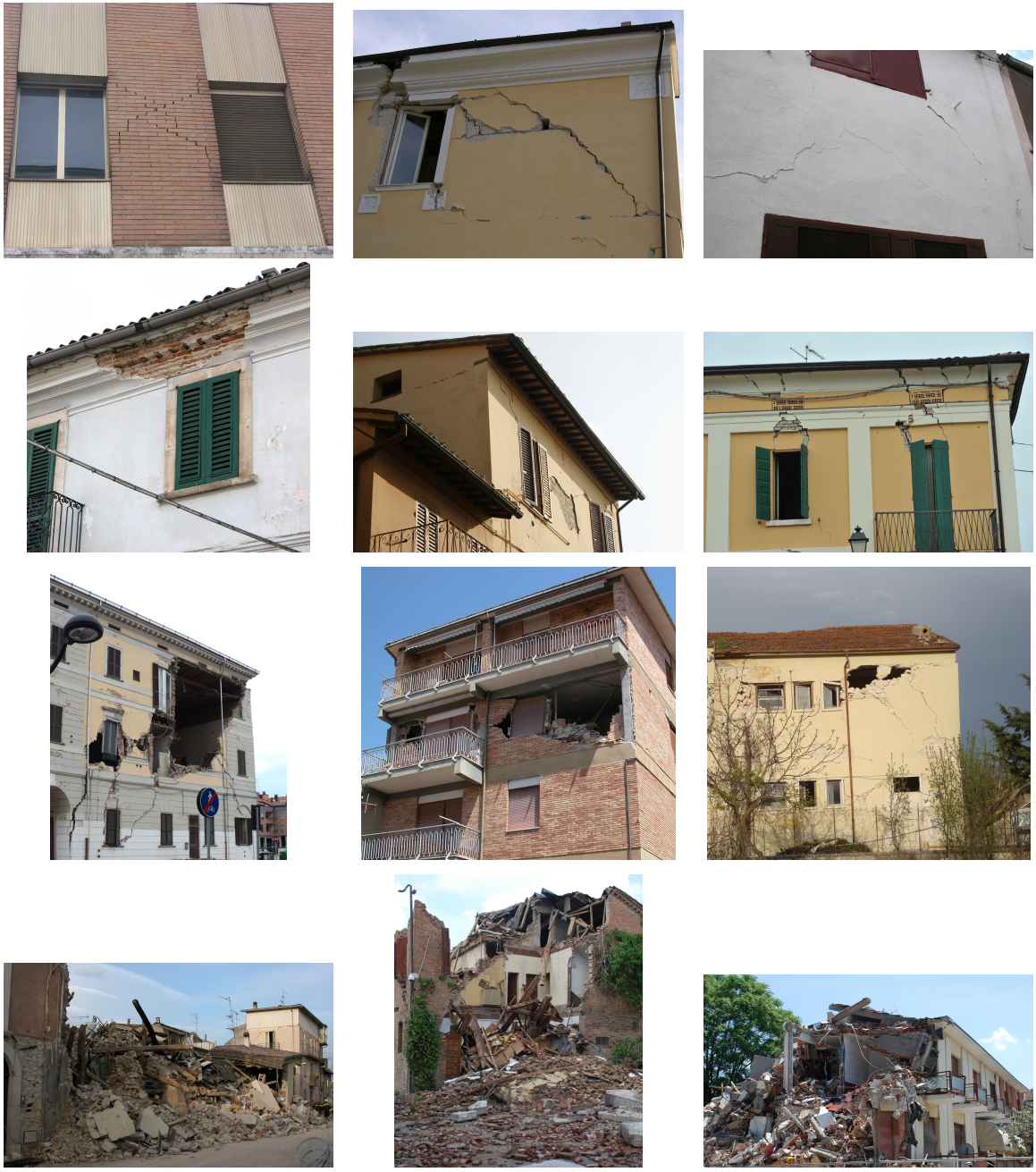
Figure 3: Sample images from the DFM test set illustrating the range of damage manifestations addressed by the MSM tool. Rows correspond to increasing EMS-98 severity, from grade 1/2 (top row) to grade 5 (bottom row), while columns reflect the heterogeneity of acquisition geometries from close-range views to mid-range façade shots and wider building-scale frames. Images obtained from the INGV Database Fotografico Macrosismico (DFM).
