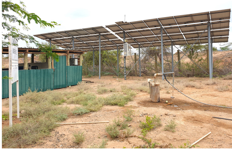
Fig 2. An example of a motorized community well site infrastructure in Turkana, Kenya, showing the well in the middle, solar panels for water pumping, and the pump control room.
