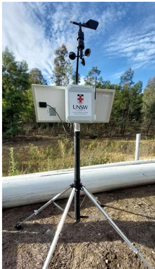
Figure 2: Deployed MOS point sensors at the mine site for continuous methane monitoring. Each metal oxide sensor was mounted on a moonlander stand capable of withstanding wind speeds exceeding 100 km/h and secured to prevent any lateral movement. Sensors were powered by rear-mounted solar panels and internal Li-ion batteries, enabling continuous operation without external backup. An anemometer installed above each unit measured wind speed and direction. All devices were geolocated, with coordinates uploaded to the cloud upon activation.
