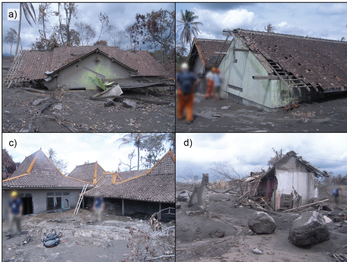
Fig. 3. Photos of slow overflow flow impacts in Bakalan village including: a) Thick deposits of up to 2.5 m partially burying houses and causing structural damage on upflow side of structure, b) inundation with minor structural damage, c) flows blocked by building fronts, resulting in little to no inundation, d) severe structural damage caused by large boulders carried by the dense flow. Photos taken 7 December 2010 by S.F. Jenkins.
