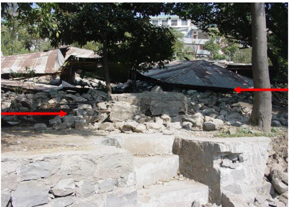
Buildings constructed using cobbles and lean mortar suffer maximum damage –Bagh AJK
