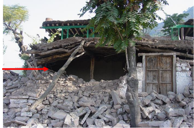
The lightweight wooden house proved earthquake-resistant compared to that constructed with blocks and improper shaped rock pieces-Dhirkot
