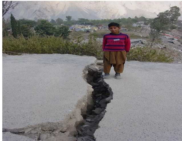
Rupture zone passing through Nisar Camp and the road site
