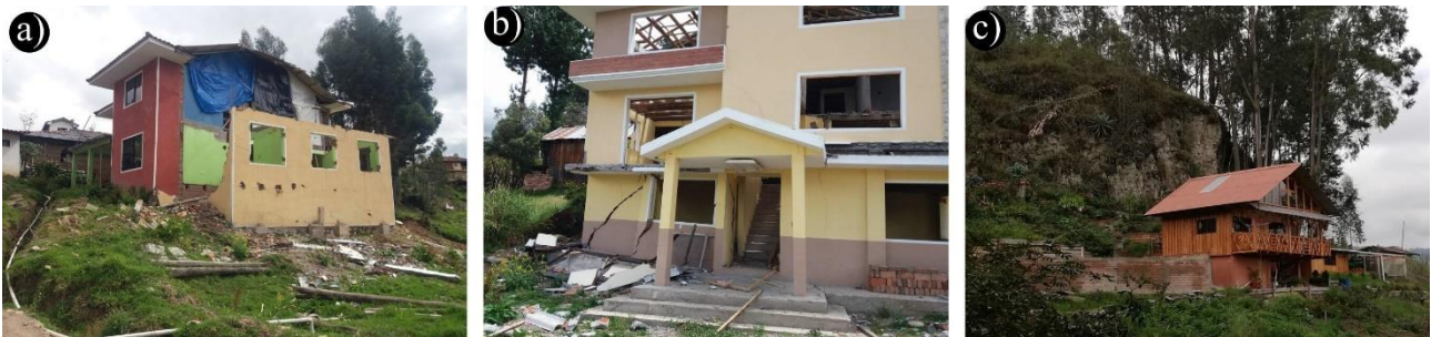
171 Fig. 2. a) House completely destroyed by a mass movement; b) house partially damaged due to a landslide; c) an 172 example of low-risk perception by the local population. The structure was built close to a sub-vertical rock wall which 173 is very prone to mass movements such as rockfalls, topples and slides (photo: M. Ramondini).
