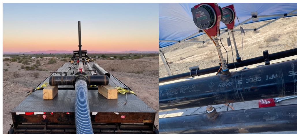
Figure 5. Metering and release trailer (left) has four pipes (0.5-inch, 2-inch, 4-inch, and 8-inch), each leading to a distinct metering location allowing a different dynamic range of release volumes. The three larger pipes used a QuadraTherm 640i insertion meter (right), with upstream 8.5 m straight run of pipe to ensure sufficient flow stabilization for all pipes. The 0.5-inch pipe was not used in this study.
