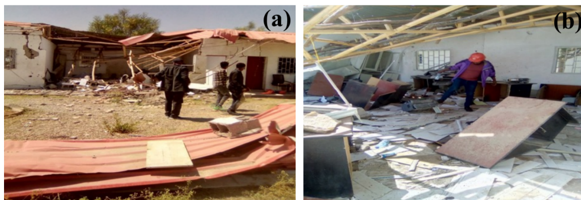
411 412 Figure 13. Damages to a) Offices and b) project documents and paper works of the Gereb Giba 413 Water Supply Development Project Office.
