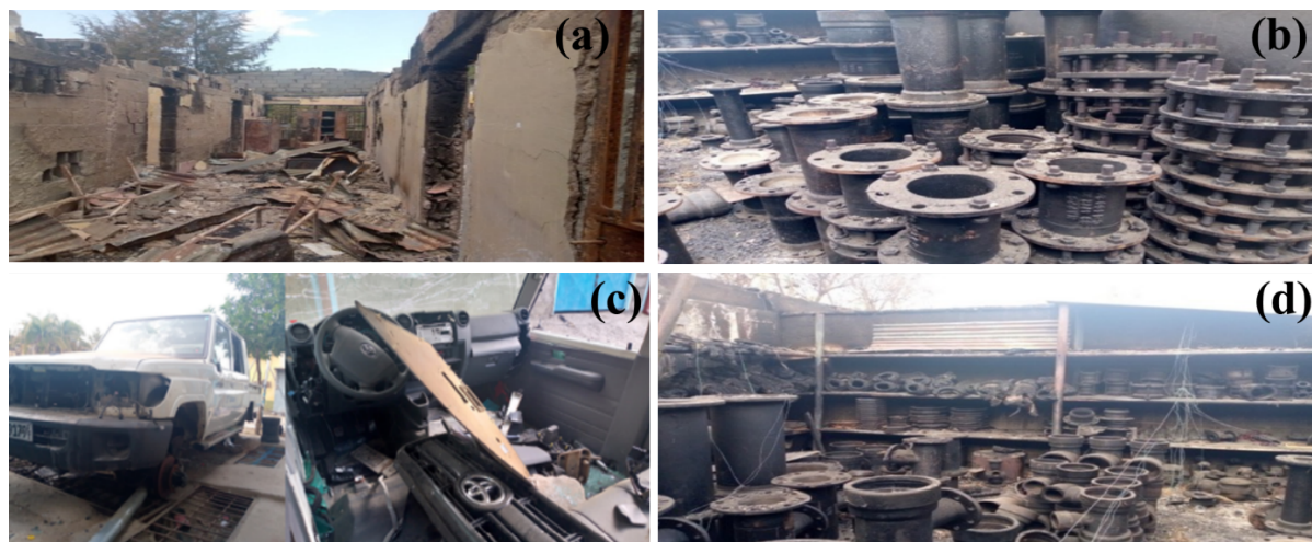
408 409 Figure 12. Damages to a) offices, b) electro-mechanical spare parts, c) office properties and 410 facilities, and d) burned electro-mechanical spare parts.
