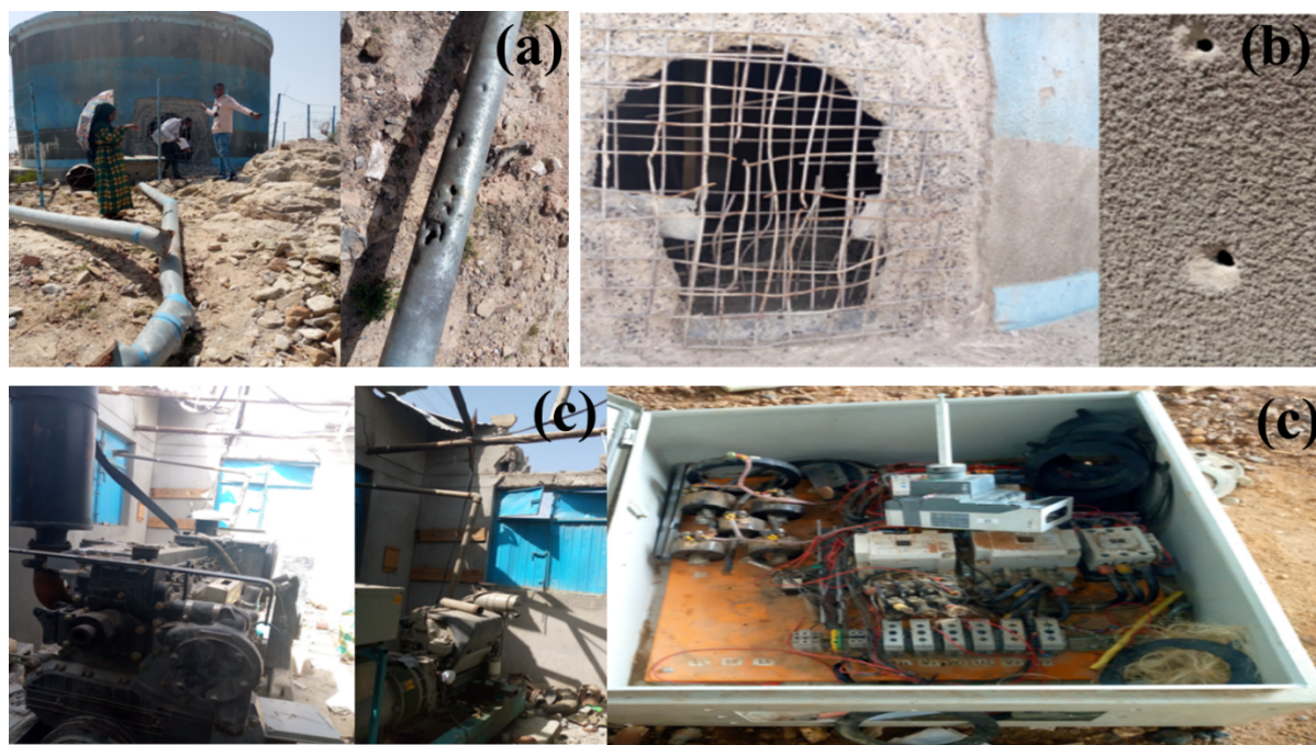
359 360 Figure 10. Damages to a) the water supply tank in Edaga Hamus (Eastern Zone), with b) 361 evidence of bullets shot into the reservoir, c) generators and d) the switchboard (control panel).
