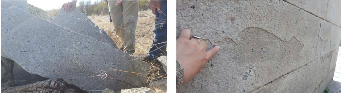
Figure 3. Left: Slab of Martinamor granite in the historical quarry. Right: Martinamor granite in the basal part of a historic building of Salamanca. Scaling in granite is common but does not affect its integrity. Explanation in Pereira 2019.
