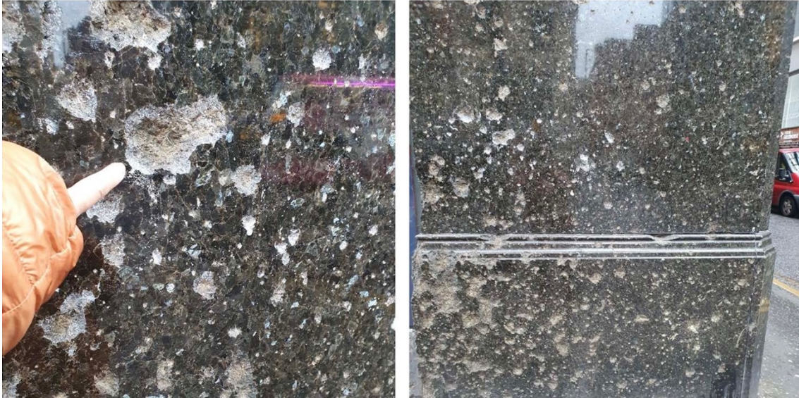
Figure 10. Bullet marks on a building façade in the center of Belfast. From the texture and observation of the stone, a syenite can be recognized. Picture by the author
