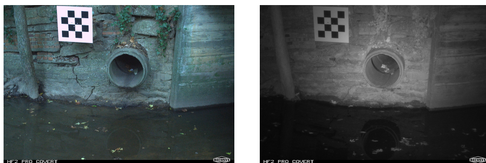
(a) (b) Fig 4. Representative images from the NC State University Softball site showing the chess board pattern panel installed above and to the left of the culvert: (a) daytime condition; (b) nighttime condition.
