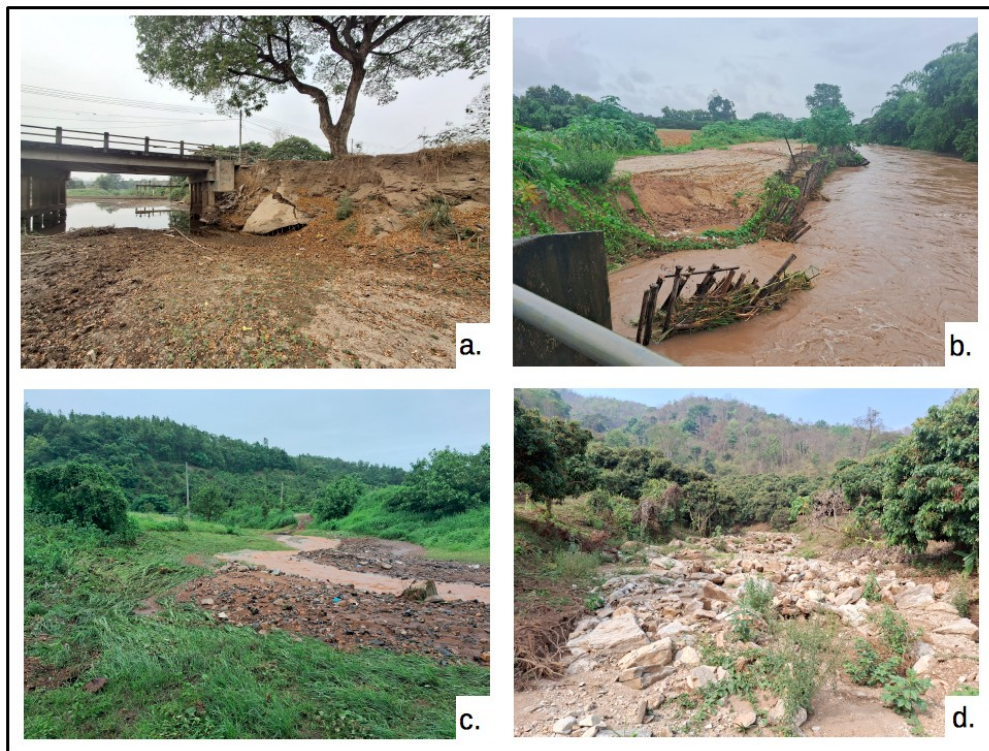
Figure 30. a. Loss of bank protection (concrete slab) and damage to a bridge in Mae Wang river; b. Loss of bank protection (wood piles), erosion and levee failure in Mae Wang river; c. Post flash flood (~4 hours) in Nam Hu river with large pebbles accumulation and record of water level in grassland. d. Debris flow in Hill 876 NE thalweg in Mae Wang (see Fig.23).
